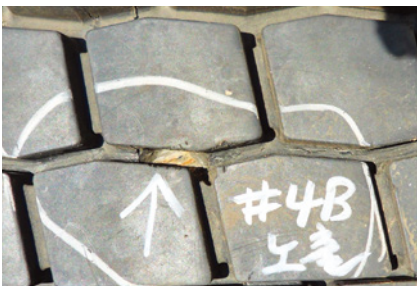
Groove Crack type 1
