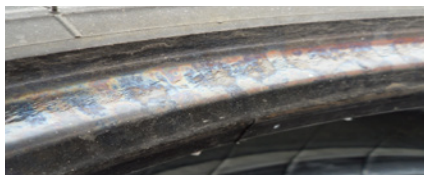
Multiple small cracks on the bead
