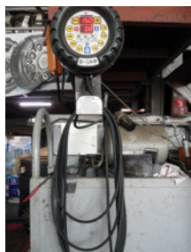
Air hose and pressure controller
